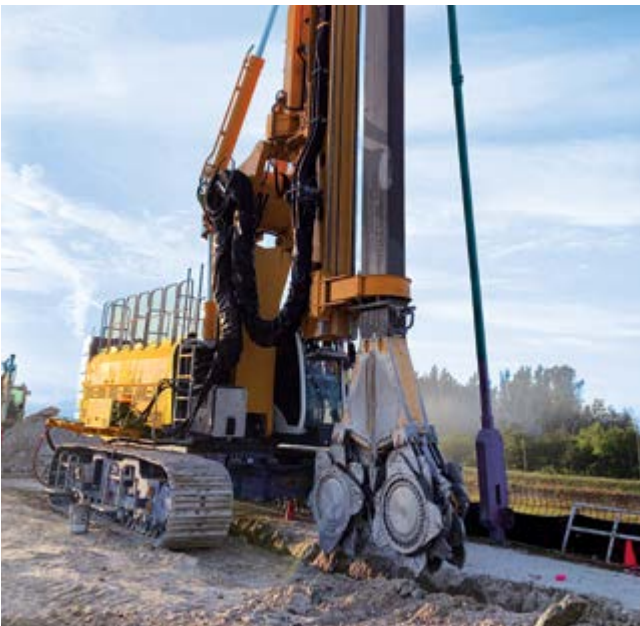
Herbert Hoover Dike, Florida, USA To improve dam security, a 28.3 km cut-off wall was installed with a depth of up to 20 m.
