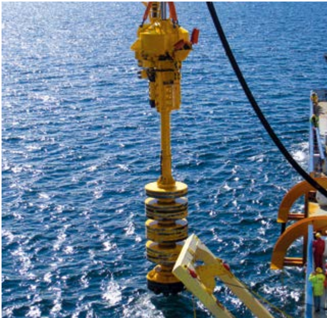
Beatrice Offshore wind park, Orkney, Scotland Foundation for a tidal turbine using a BSD 3000 seabed drill.
