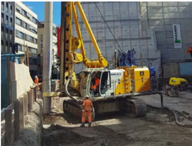
New construction of office building, Munich, Germany Execution of secant pile wall with a diameter of 620 mm and depth of 18 m using the FoW method.
