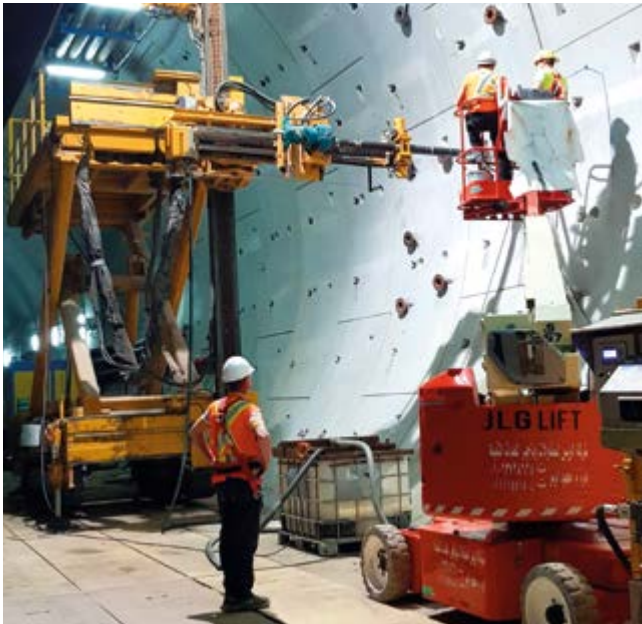
Tunnel under Suez Canal, Ismailia, Egypt Construction of four cross slats to connect two roadway tunnels with brine freezing.
