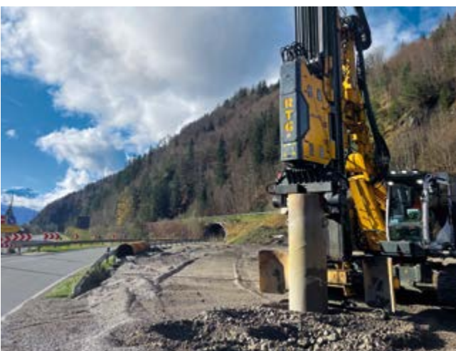
New construction B2, Eschenlohe, Germany For the new B2 bypass, a total of 6,200 m of vibro textile columns were constructed.
