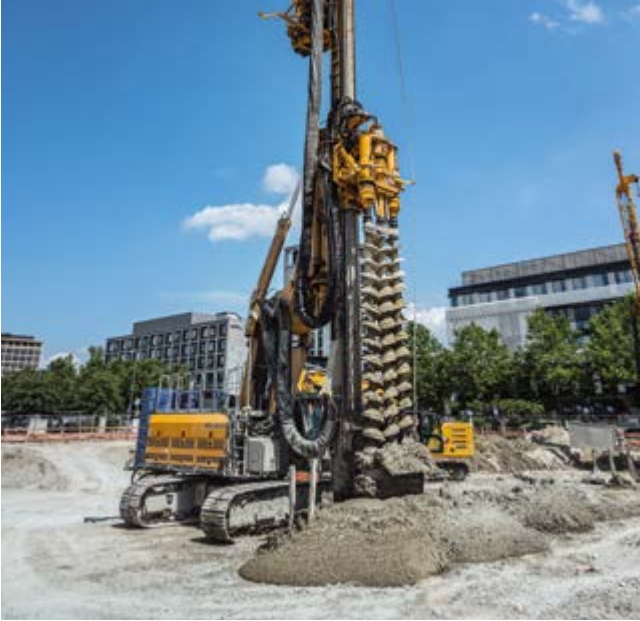
Parkstadt Schwabing, Munich, Germany Construction of a 6,000 m 2 single-anchored Mixed-in-Place cut-off wall for a 9 m deep excavation pit.
