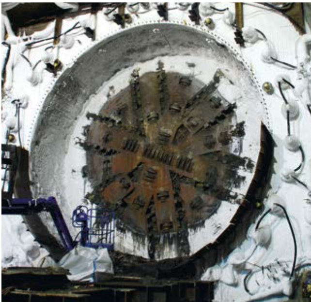
Üsküdar Metro Station, Istanbul, Turkey Construction of 33 horizontal freeze pipes and twelve thermometer pipes using nitrogen freezing.
